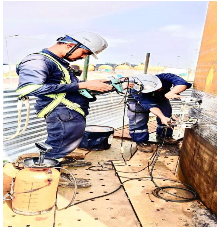
PAUT/ToFD Inspection of Mounted Bullets at Vijay Tanks & Vessels, HRRL, Rajasthan, India
